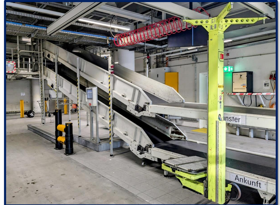
Sorting luggage area at Munich Airport, November 2024
